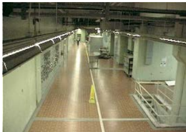
Figure 6 - New generator floor
