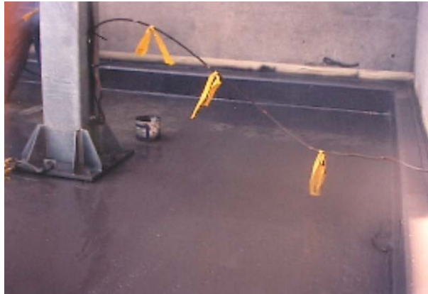
Figure 13 - Transformer bay oil containment liner
