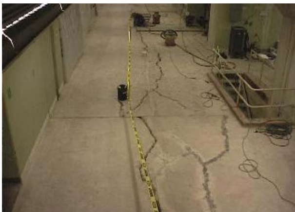
Figure 5 - Tile and mortar bed removed exposing extensive cracking of underlying concrete
