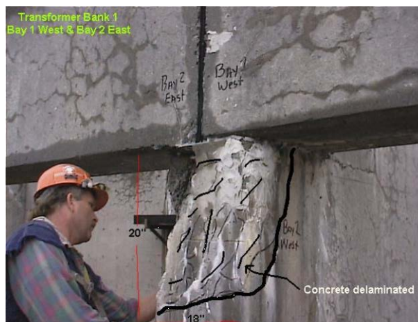
Figure 14 - Beam bearing area delaminated concrete
